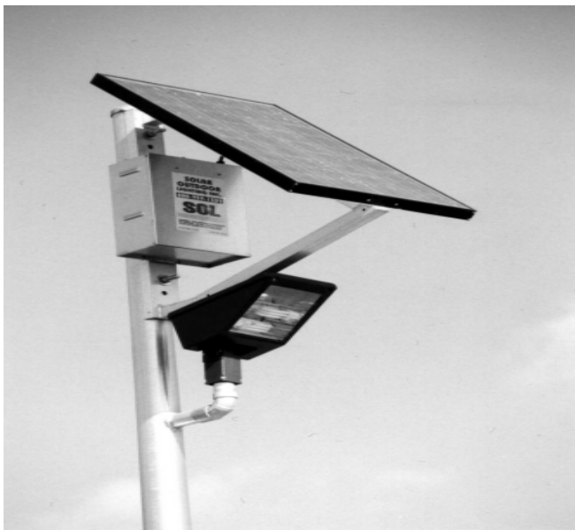
Solar lights at the Overland Park Golf Course parking lot
