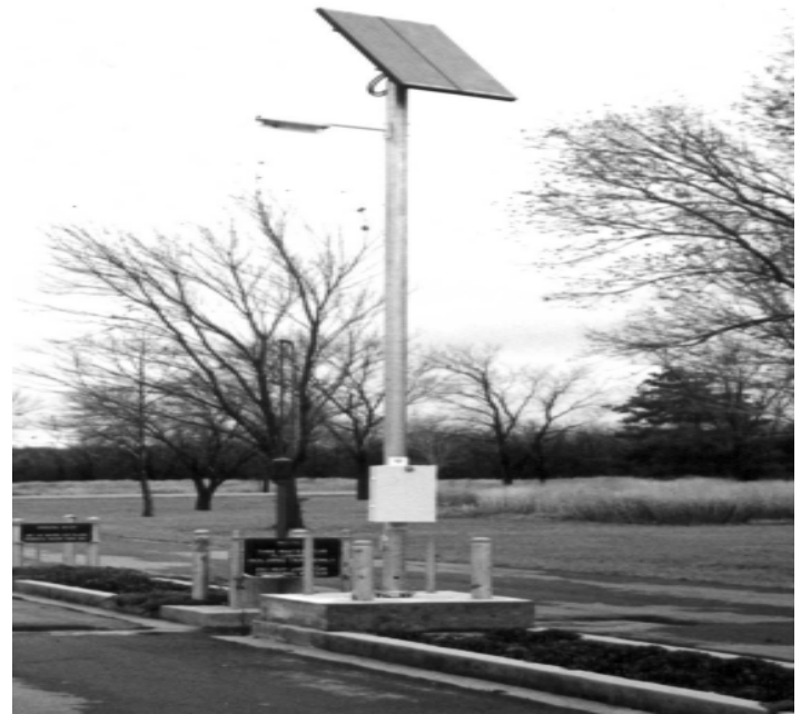
Solar lighting is used to illuminate the pumping station at Pomona State Park
